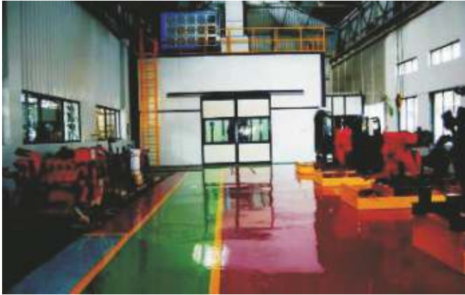
New state-of-the-art acoustic guard testing and packaging facility for FMUL fire fighting pumpsets at Kirloskarvadi
